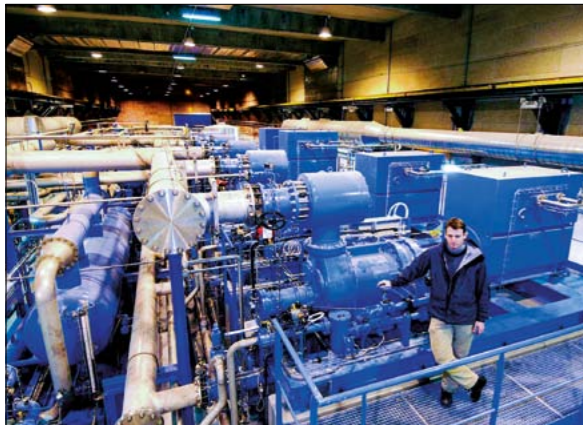
Fig. 2. The compressor unit of the 4.5 K refrigerator at Point 6. The unit provides 18kW cooling capacity. There are eight of these units in the complete system.
